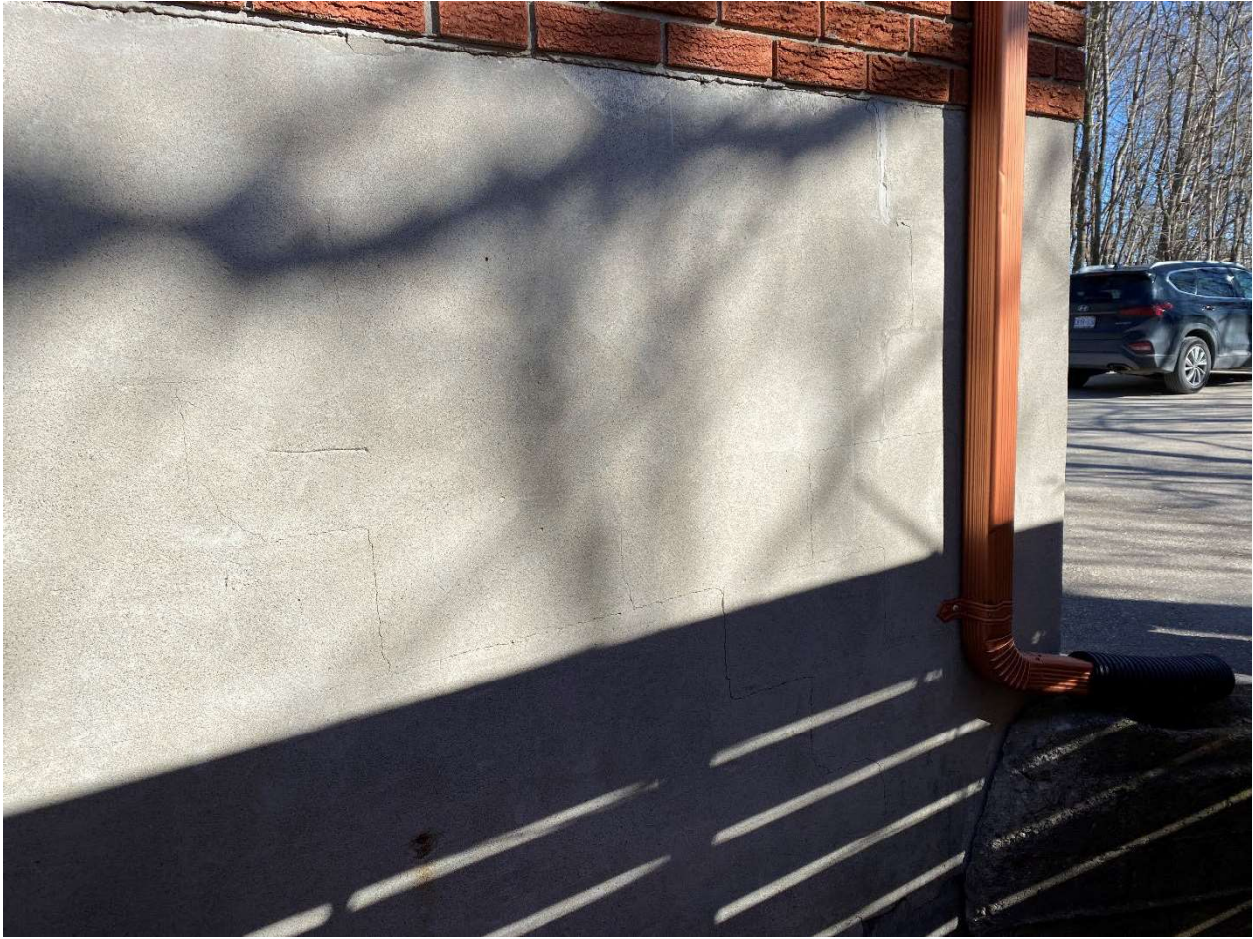
Photo 4: Cracks in South Foundation Wall
