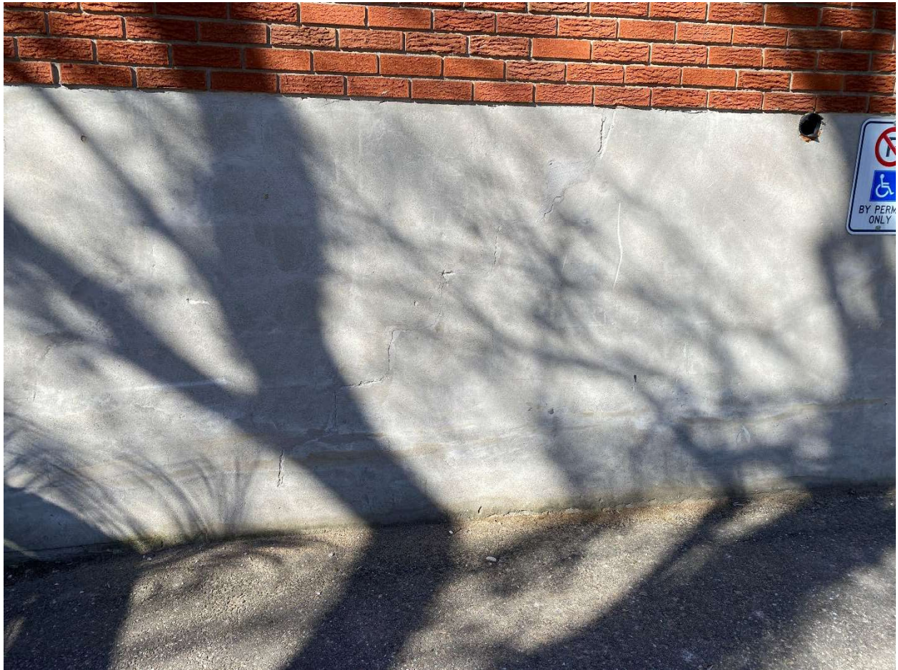
Photo 3: Step Cracks Near South End of East Foundation Wall
