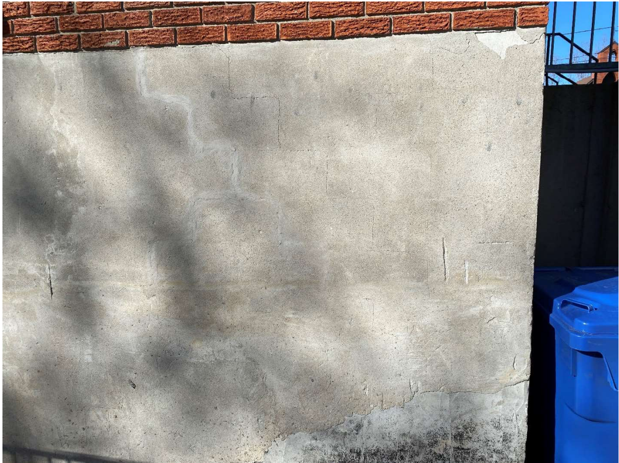
Photo 1: Step Cracks Near North End of East Foundation Wall
