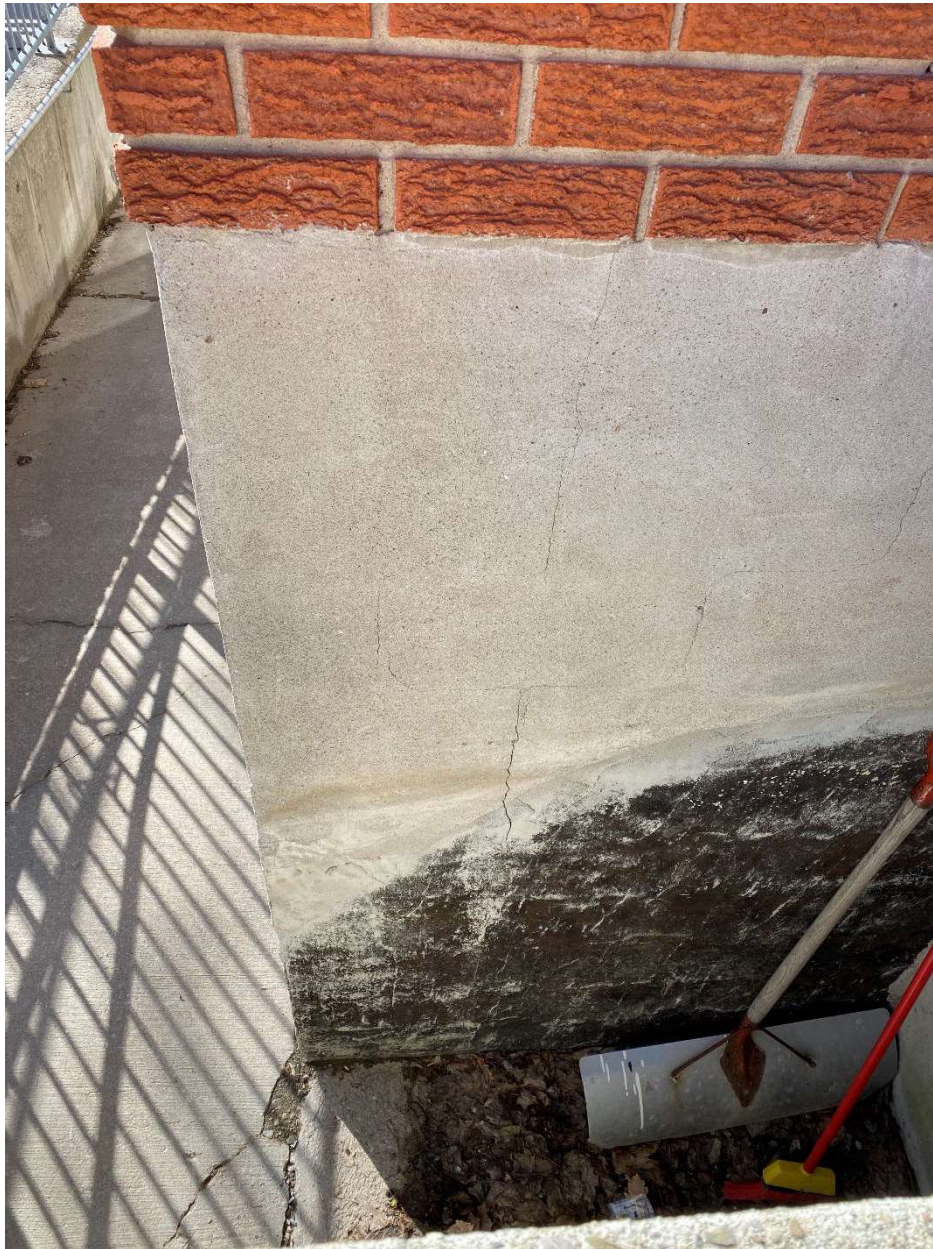
Photo 5: Vertical Crack in North Foundation Wall
