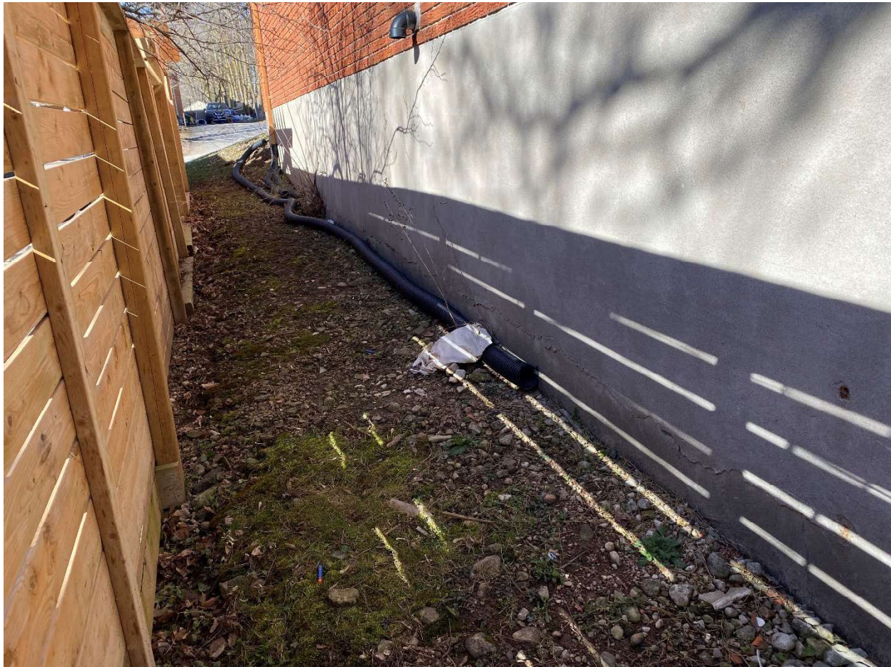
Photo 6: Downspout and Sump Pump Outlet Directed Against South Foundation Wall
