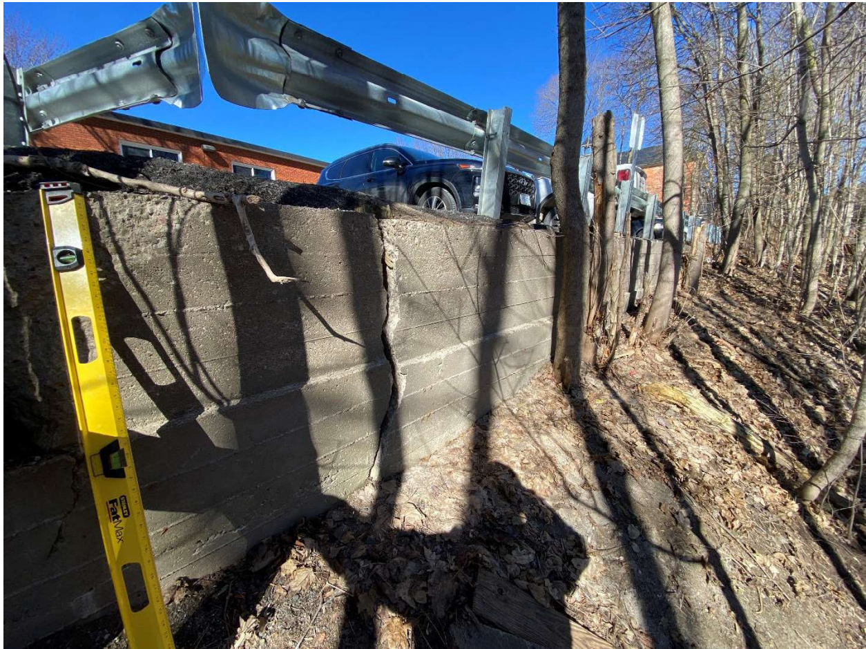
Photo 9: Crack Near Southeast Corner of Retaining Wall
