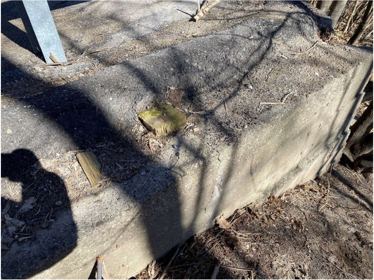
Photo 8: Wood Post Stub
